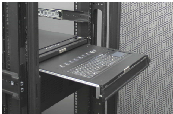
Figure 6. Pushing the upper LCD drawer until it is located in the rack.
